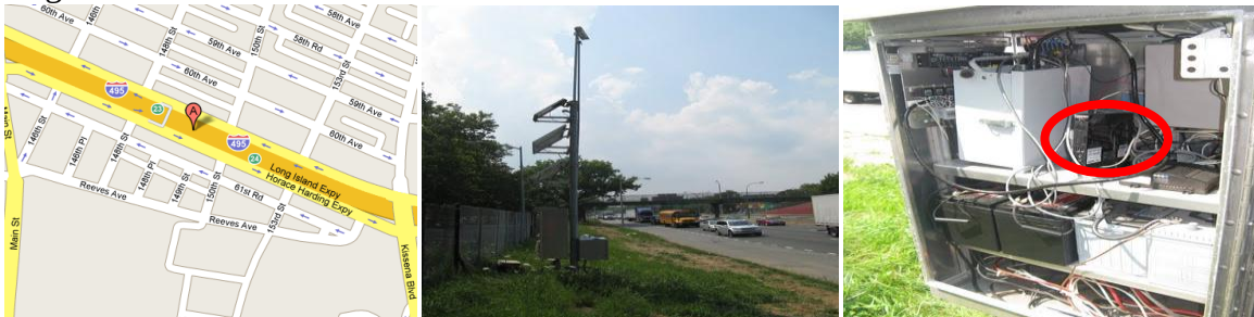
FIGURE 3: Installation in New York. The red oval indicates the video processor.
