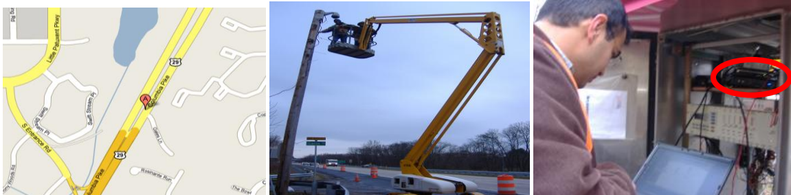
FIGURE 2: Installation at Maryland. The red oval indicates the video processor.
