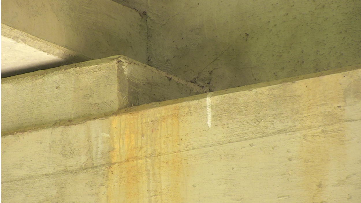
Figure 5.22: Hairline cracking observed with the drone.
