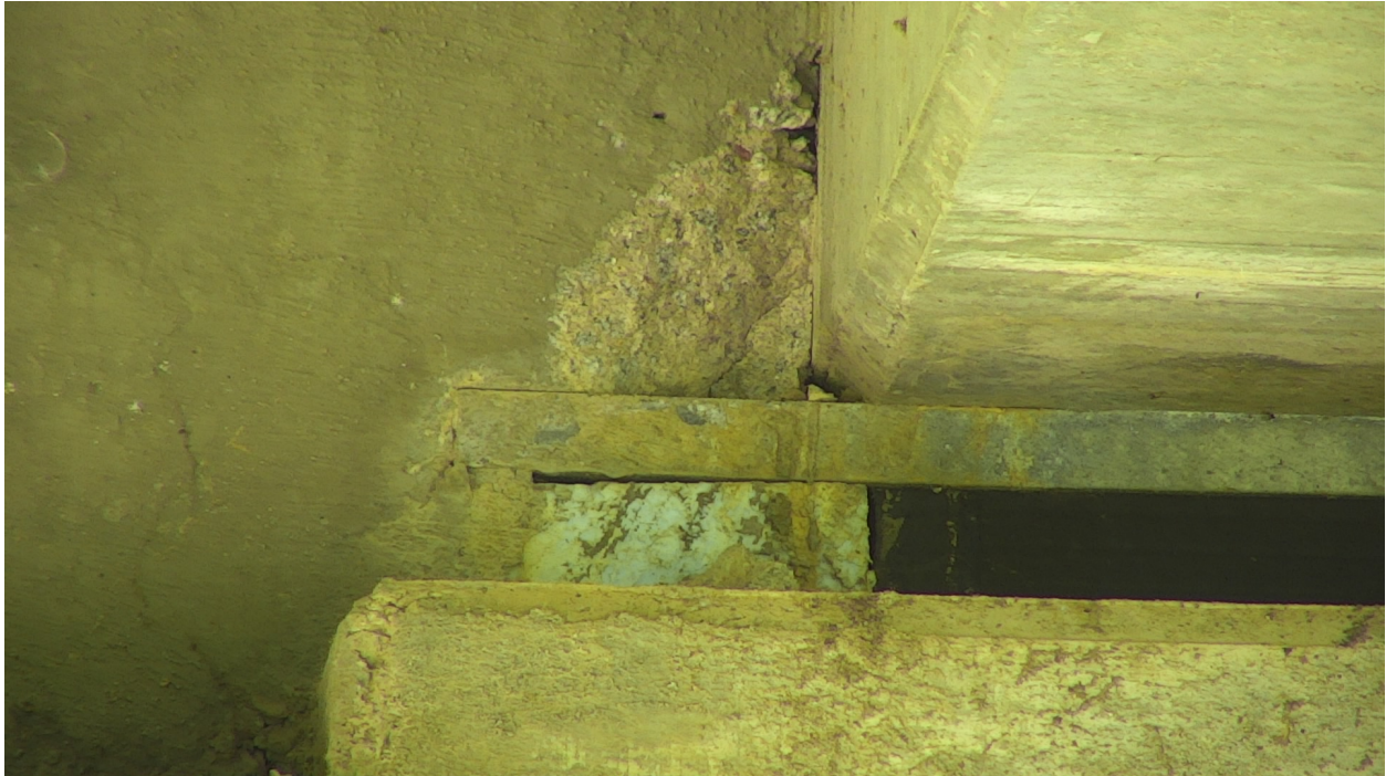
Figure 5.20: Bearing unable to see sufficiently #1.
