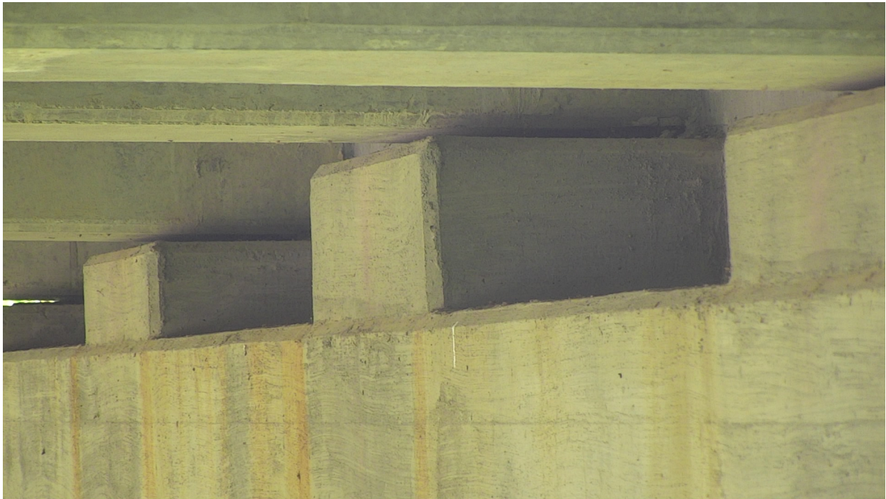
Figure 5.21: Bearing unable to see sufficiently #2.
