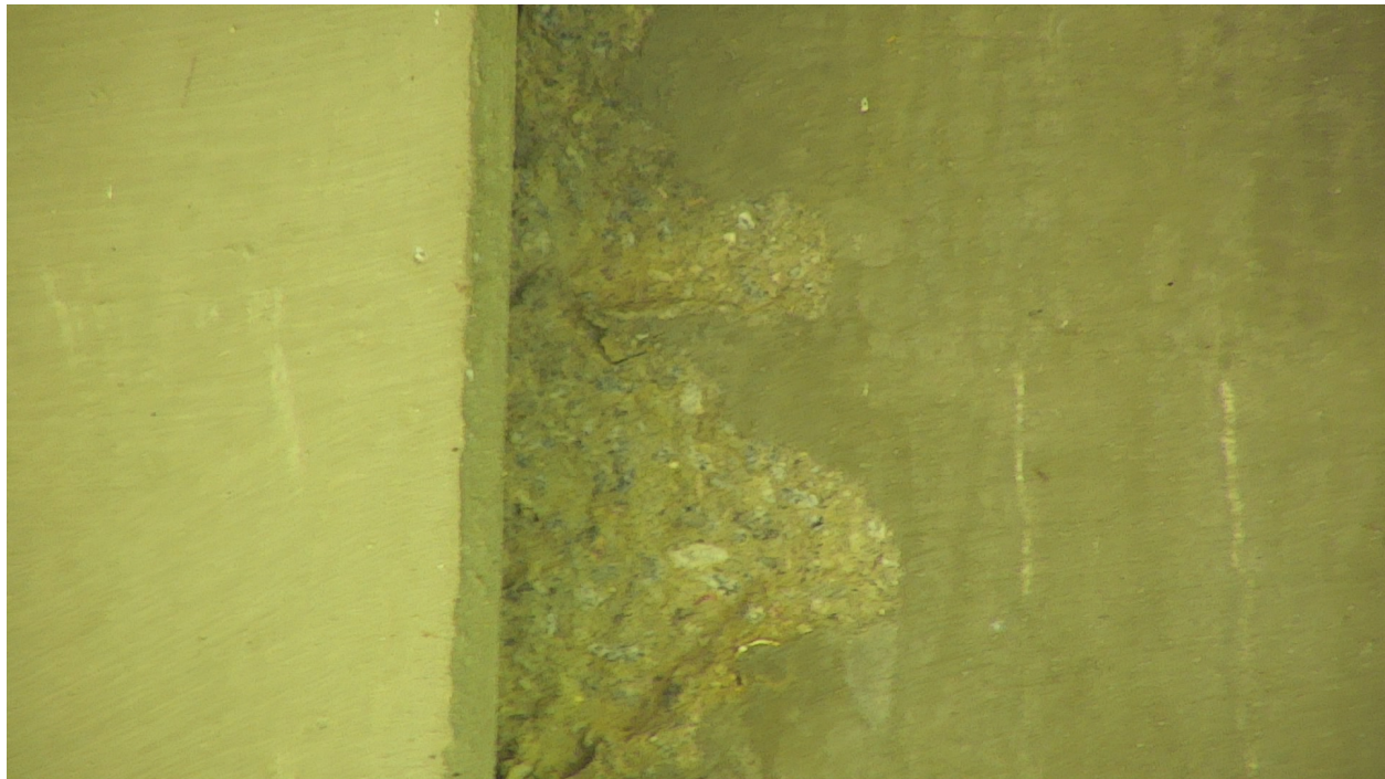
Figure 5.25: Minor spalling observed with a drone.
