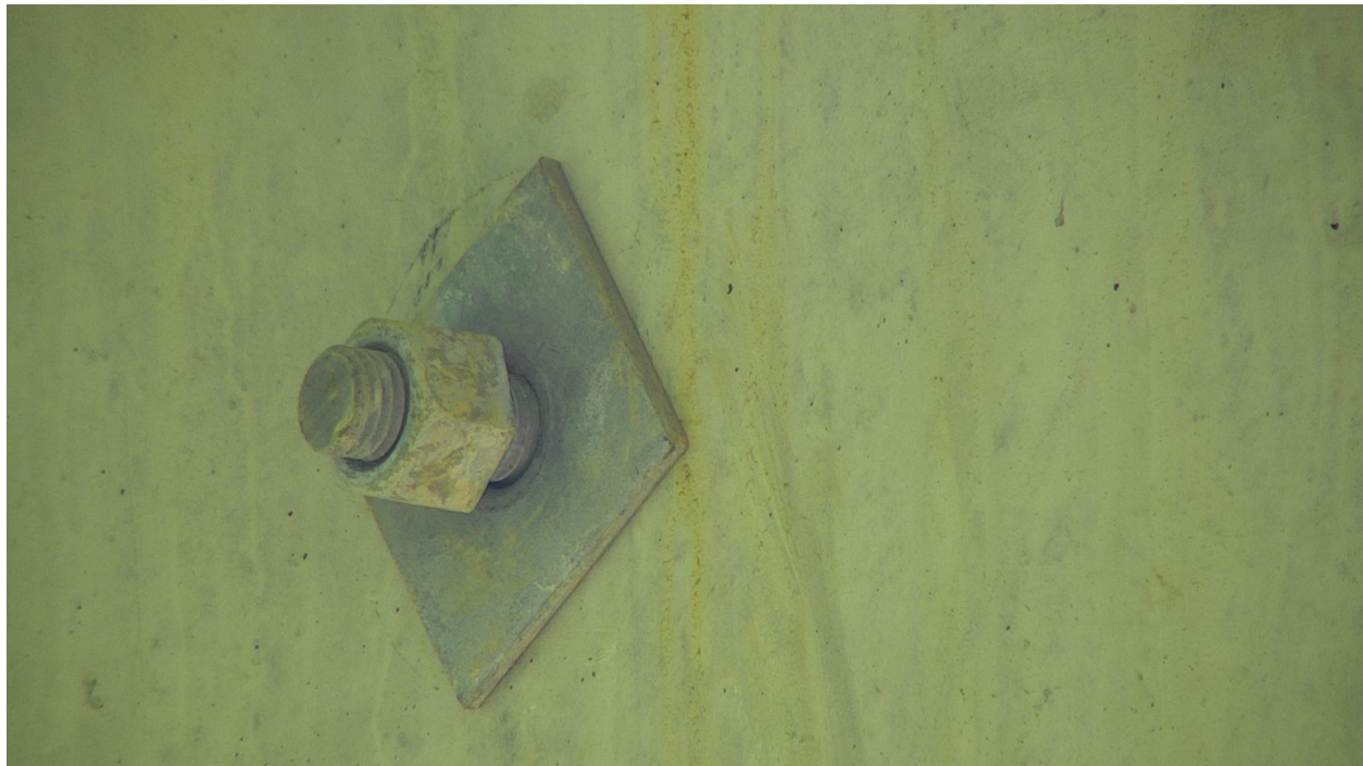
Figure 5.24: Anchor bolt not tightened down.
