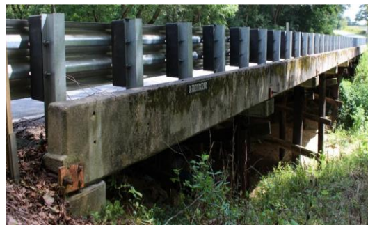
Figure 3-0-7: The two lane bridge (S-97) over Johnson Creek near Abbeville, SC: actual bridge
