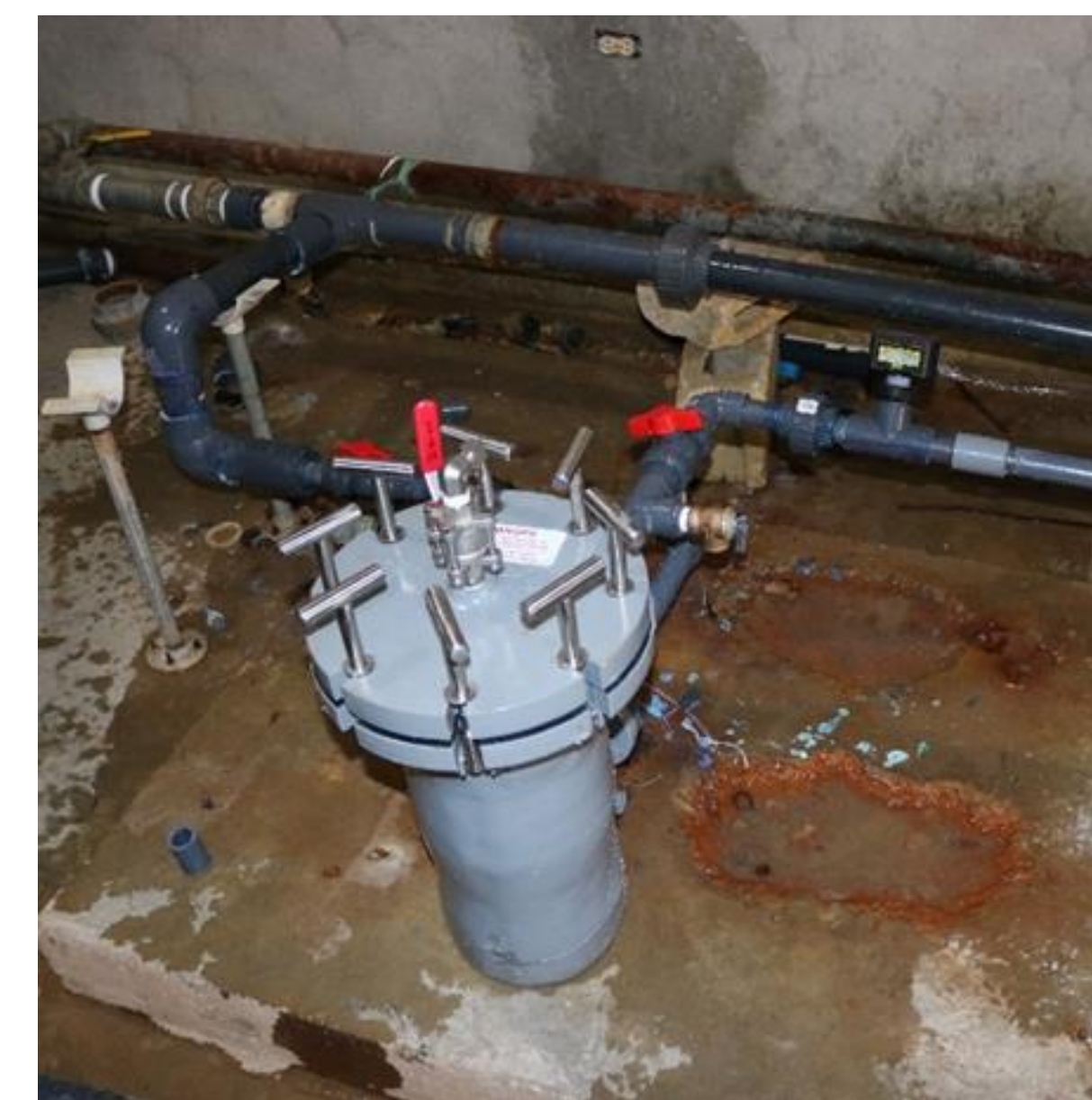
Figure 3. The newest chlorinator in the Cange Municipal Water System installed in March of 2018.
