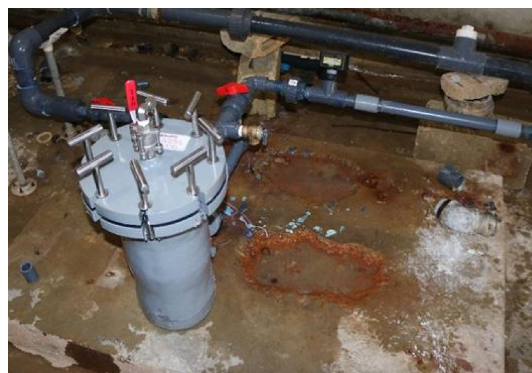
Figure 4. The newest chlorinator in the Cange Water System installed in March 2018.
